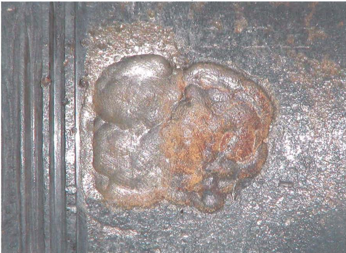
Figure 10 Close-Up of the External Corrosion on Section #4
