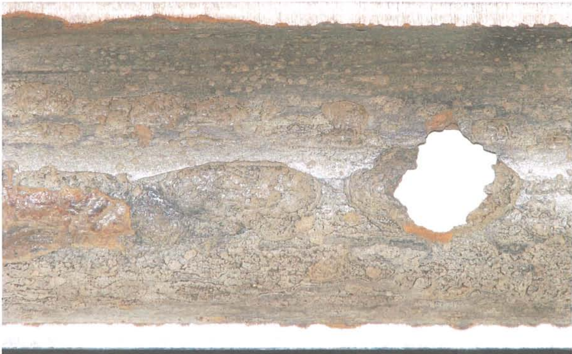
Figure 6 Internal Corrosion on Section #2
